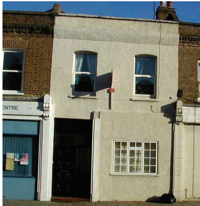
Bad Practice: Fascia sign removed
